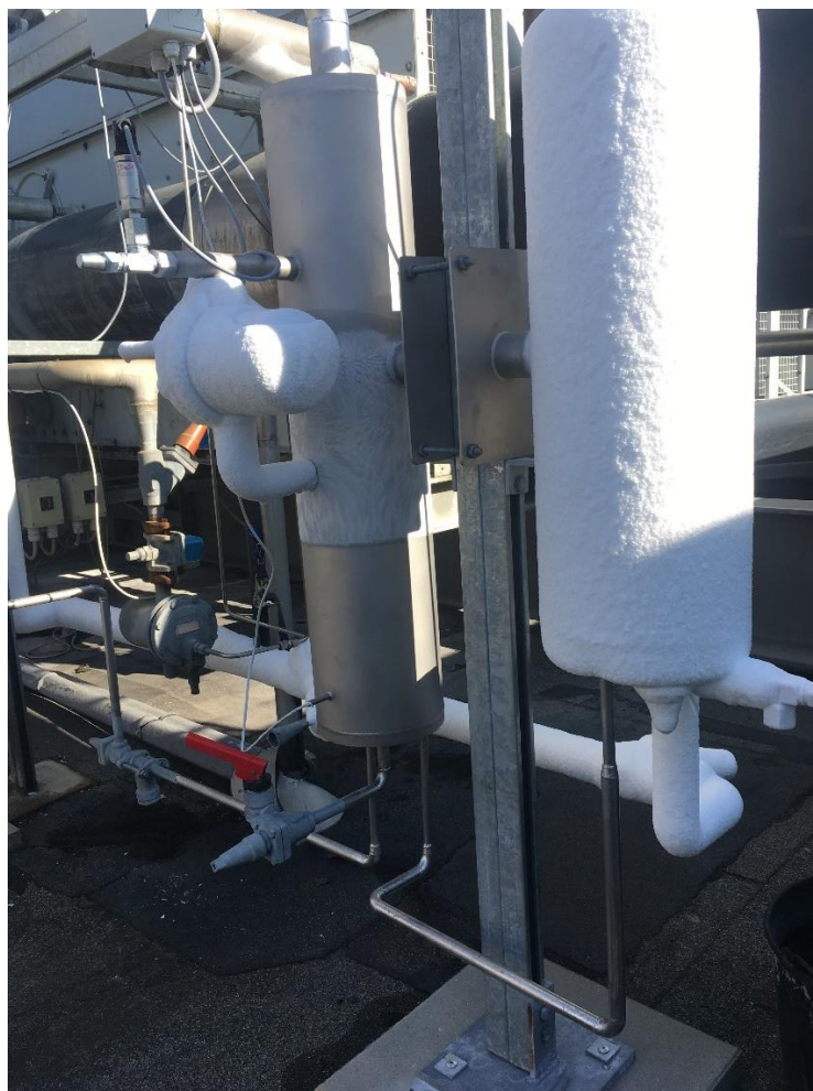
CPW ready to drain for water and sludge separated from system.
