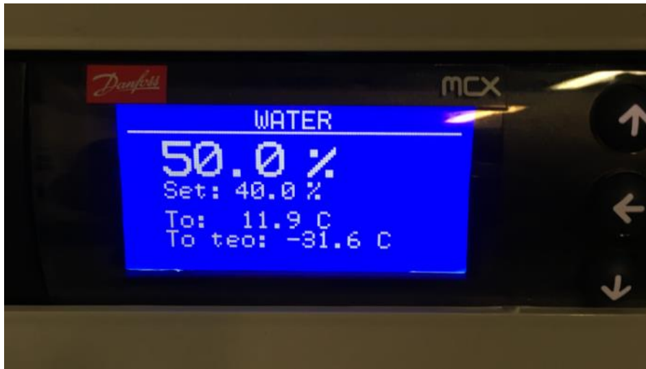
CPAC Controller showing high water content in CPW12. Water draining necessary.
